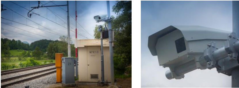
Figure 2. LiDAR sensor installed at the level crossing.
